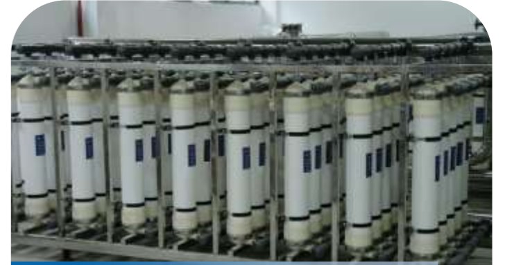
CHINA - BOILER FEEDWATER 3420m 3 /d - UFH-PSS1060
