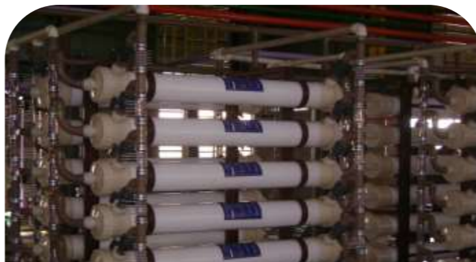
GERMANY - WINE CLARIFICATION 2015m 3 /d - UFH-PST8060
