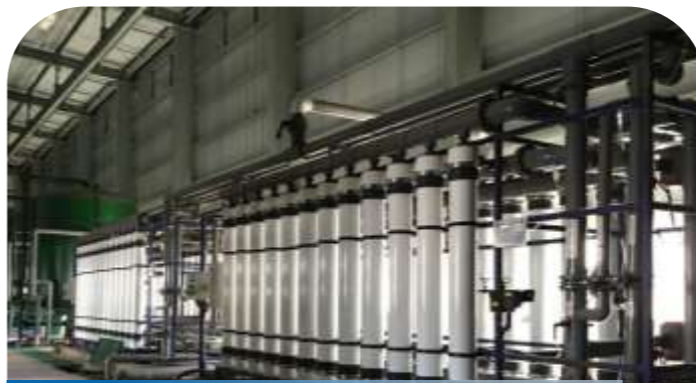
CHINA - LAKE WATER PURIFICATION 7000m 3 /d - UFP-2880
